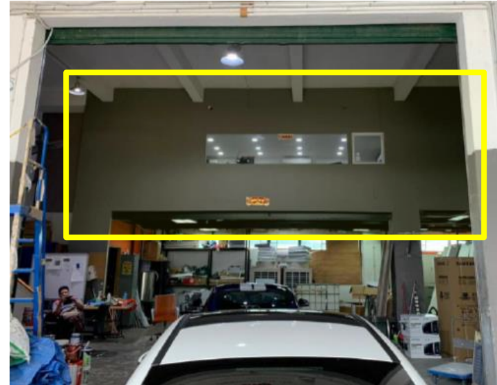
Mezzanine works without approval of plans
