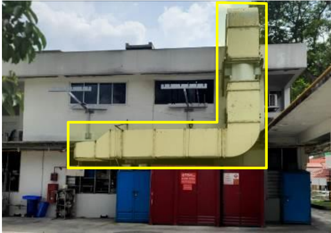
Installation of Kitchen Exhaust Ducting without approval of plans
