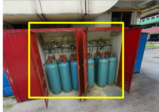
Installation of LPG Manifold without approval of plans
