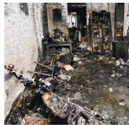
The aftermath of a fatal fire at a flat in New Upper Changi Road in March 2022. Preliminary investigations showed that the blaze started from a personal mobility device charging in the living room of the fourth-storey flat. ST FILE PHOTO
